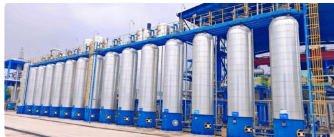
The World's highest-pressure PSA hydrogen extraction unit
