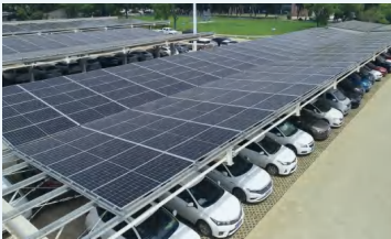
"Photovoltaic power-energy storage-Battery charging zero-carbon emission unit" charging station
