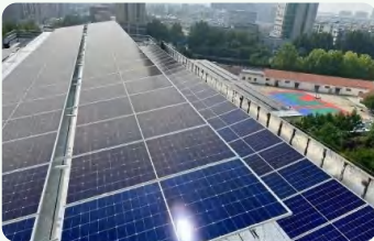
Rooftop photovoltaic modules
