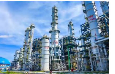
Distillation system of Quanzhou Petrochemical
